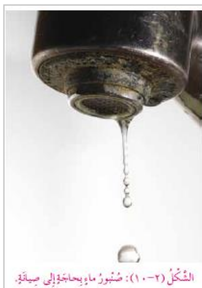
(Figure 2-10): A tap in need of repair.
